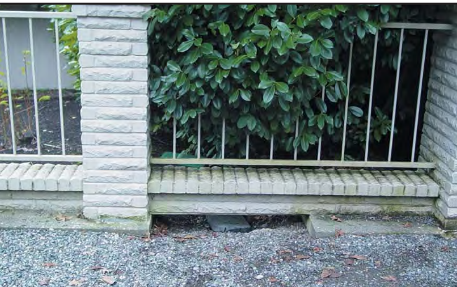
Meter is located underneath the fence
